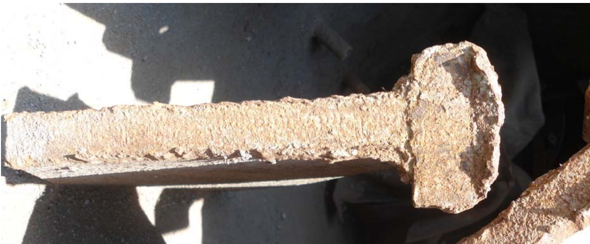
Photo 2, 3 & 4: most of the welds shown are without fusion of the gussets. The weldment is not seen to the gussets. When the weld is properly fused, metal will be seen pulled out in a haphazard manner. The edge preparation is supposed to be with hardly any land as per IBR regulation / BS code.
