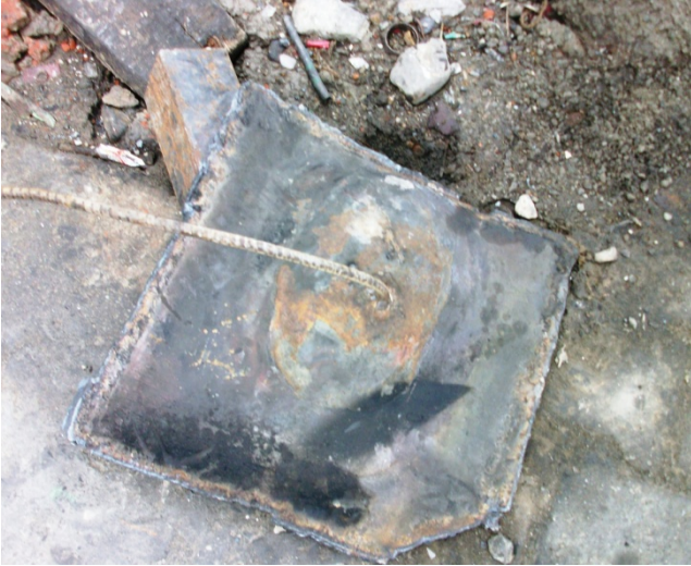
Photo 1: The part of the furnace shell that bulged second time.
