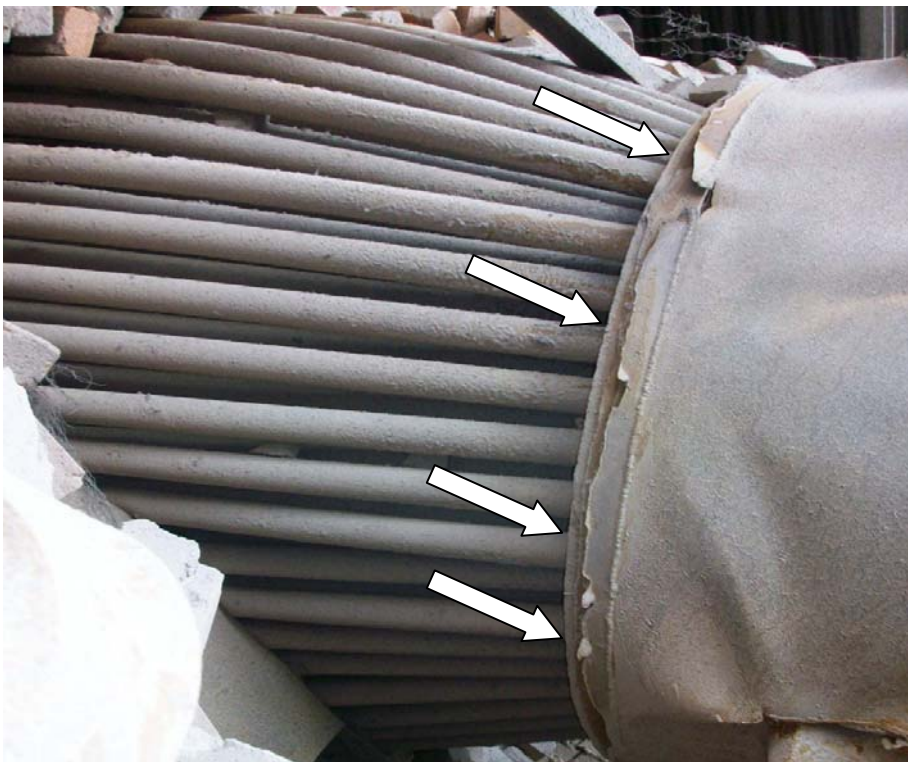
Photo 1: It is seen that the tube sheet to shell weld is not torn off even a bit. This can happen if the fusion was not proper.
