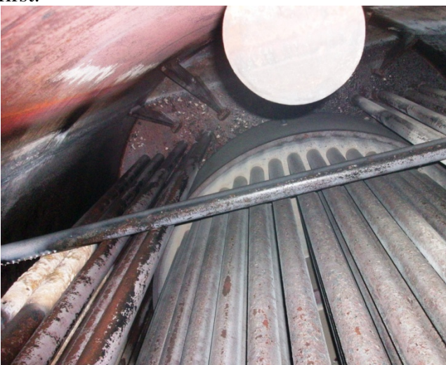
Photo 5: water side showing small amount of scales.
